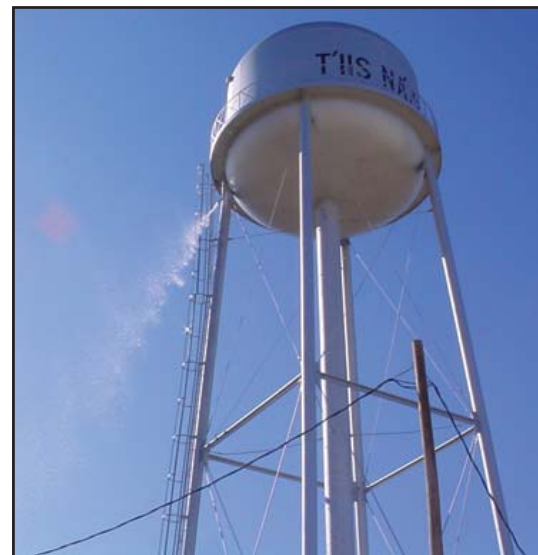
The lack of an automatic shut off valve for the water tower at T'iis Nazbas Community School in Arizona causes periodic overflow until it is manually shut off.
