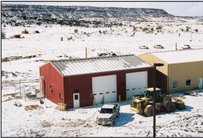
A fire station at Low Mountain is now under construction next to Jeehdeez'a Academy's new replacement school and will soon join the six fire stations that have recently received their certificates of occupancy.
