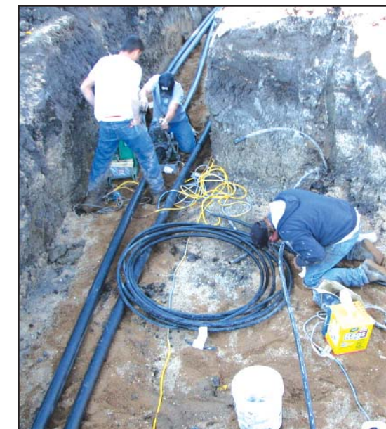
Last year, workers at Circle of Nations - Wahpeton Indian Boarding School (above) fused high density polyethylene piping running through a trench that is now covered over.
