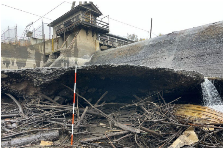
Wapato Diversion at Wapato Irrigation Project, Washington – scour hole
