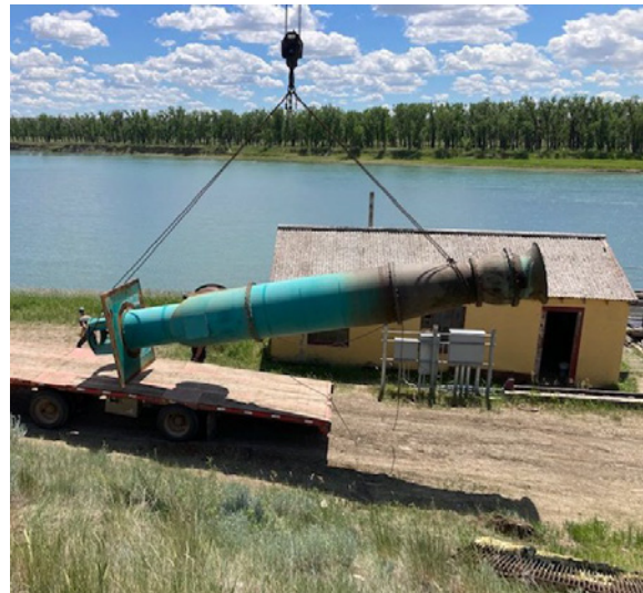
Wiota Pumping Plant at Fort Peck Indian Project, Montana – removal of old pump set for refurbishment.
