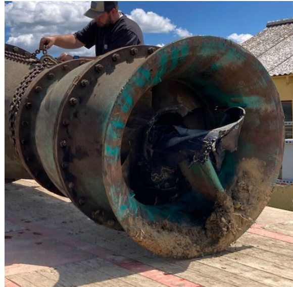
Wiota Pumping Plant at Fort Peck Indian Project, Montana – belt wrapped around impellar.
