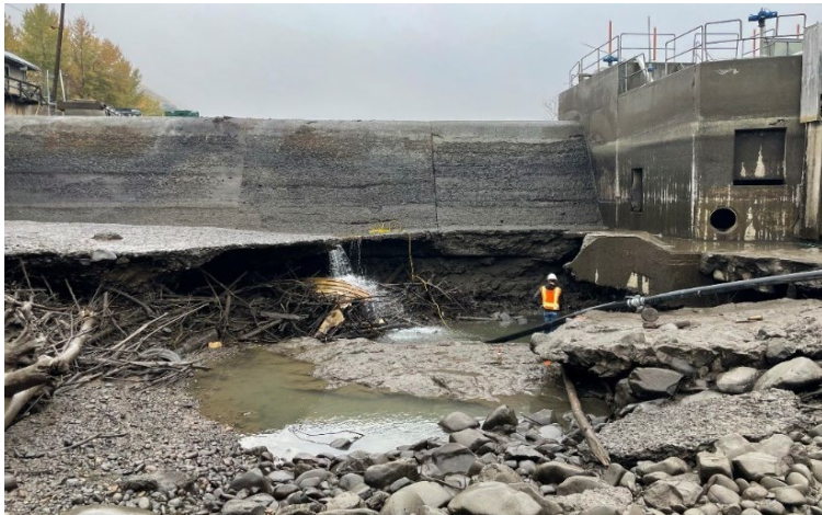
Wapato Diversion at Wapato Irrigation Project – scour hole
