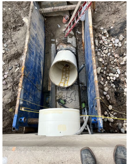
Portneuf Pumping Plant at Fort Hall Indian Irrigation Project, Idaho – rehabilitation work in progress.
