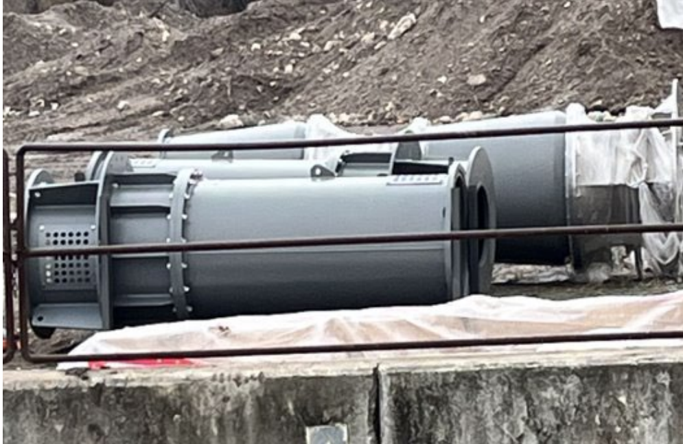
Portneuf Pumping Plant at Fort Hall Indian Irrigation Project, Idaho – new pumps ready to install.
