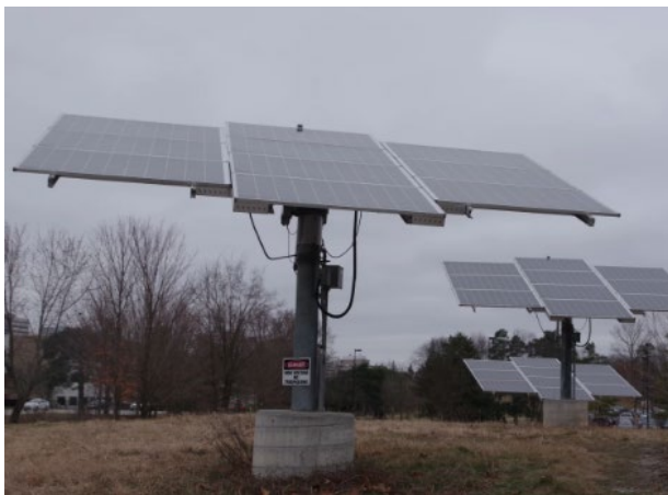
Solar Array at the Gun Lake Tribe Reservation, Michigan.
