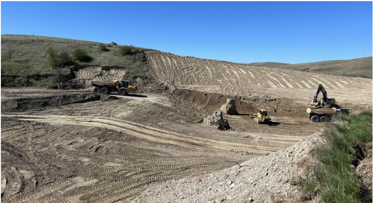
Oglala Dam from the top of the dam looking into the spillway excavation
