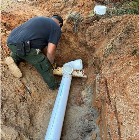
Installation of wet system that conveys harvested rainwater to the storage tank
