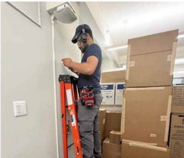
Wi-Fi installation in museum collection space
