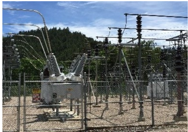
Kerr Substation, MT
