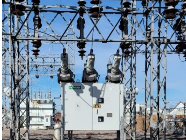
Transmission breaker at Coolidge Substation, AZ
