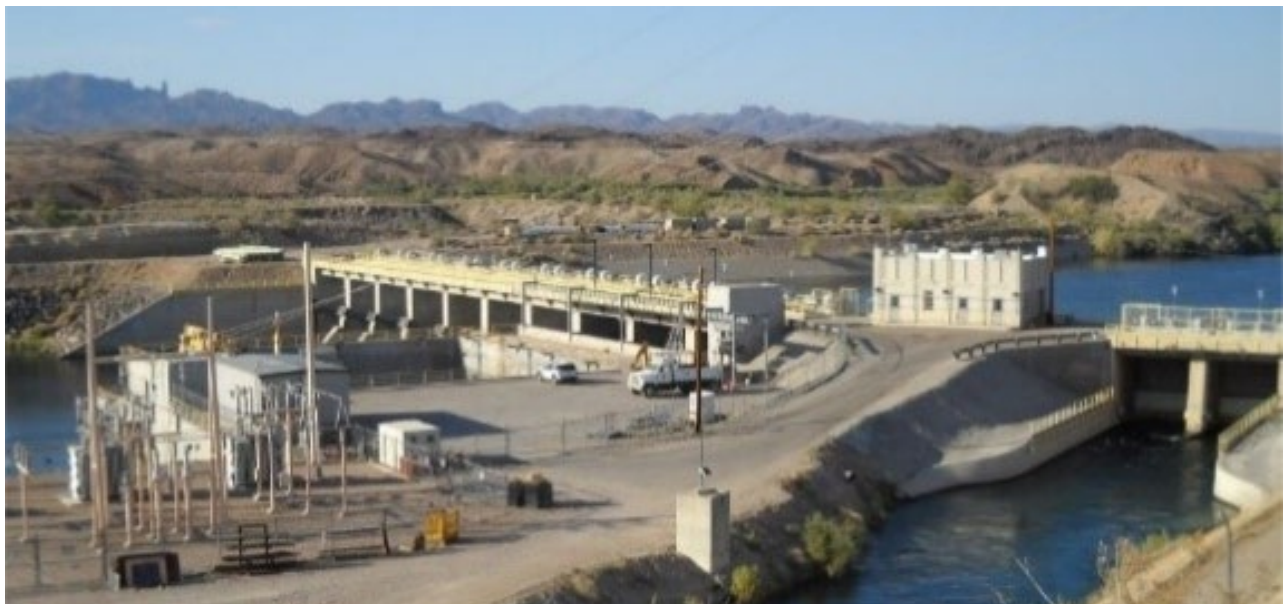
Power Generation Facility at Headgate Rock Dam, AZ/CA border
