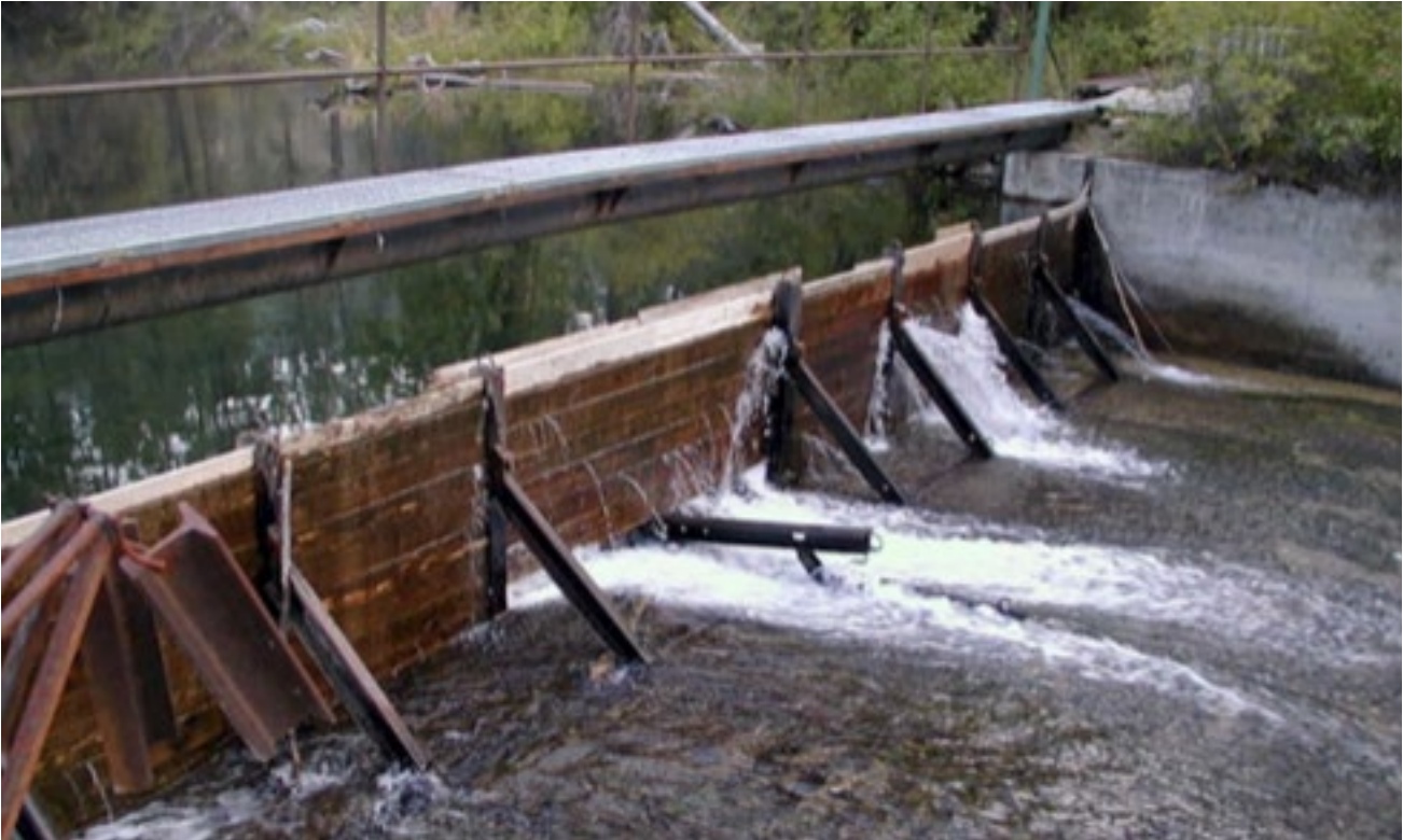
Diversion Dam before replacement—Jocko K Diversion at Flathead Indian Irrigation Project, Montana
