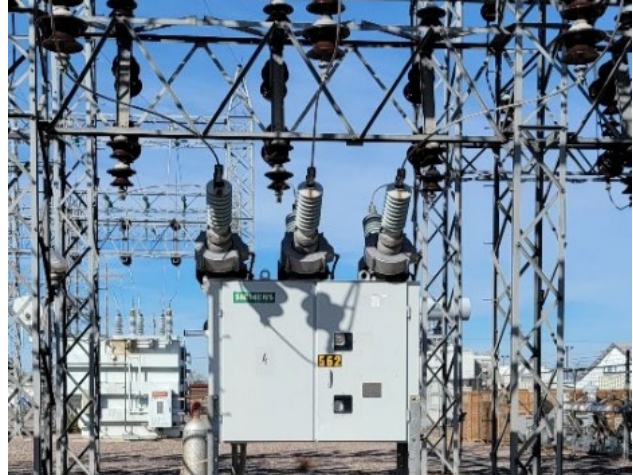
Transmission breaker at Coolidge Substation, AZ
