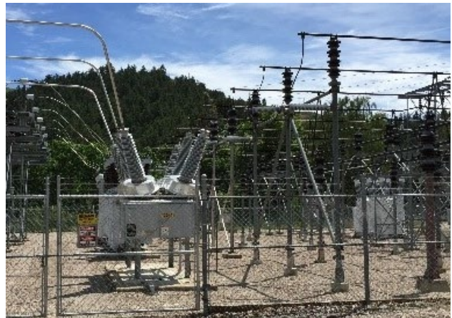
Kerr Substation, MT
