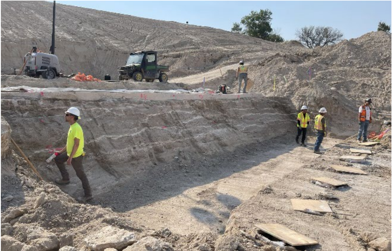
Exposed bedrock near the bottom of the excavation for the new spillway at Oglala Dam; placing the first layer of concrete for the new spillway at Oglala Dam
